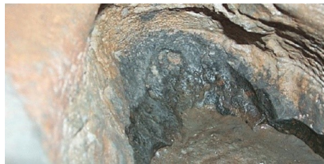
Davis-Besse corrosion | NRC
